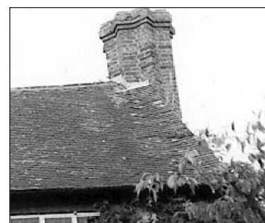
A variety of chimney types can be found, mainly brick built and sometimes of an intricate style.
