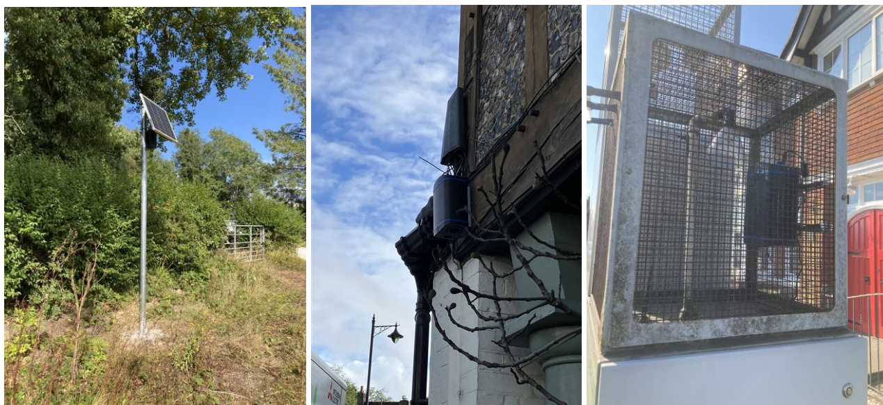
Figure C.4 – Air Quality Sensors installed in Horsham
