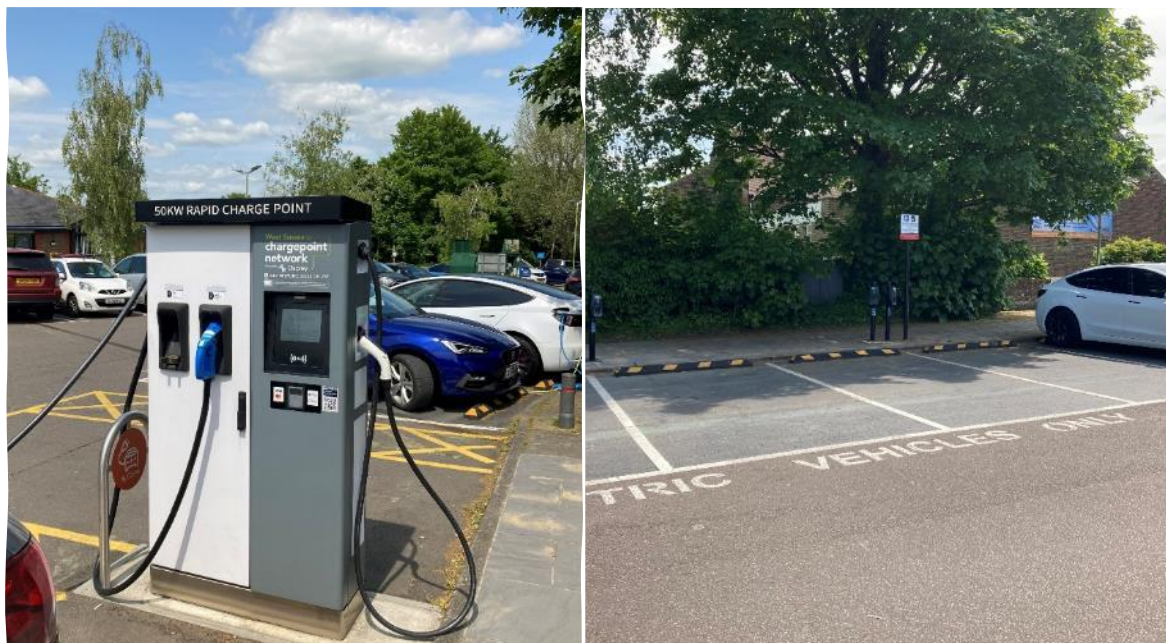
Figure 2.4 – Electric Vehicle charging point at Storrington Library car park
